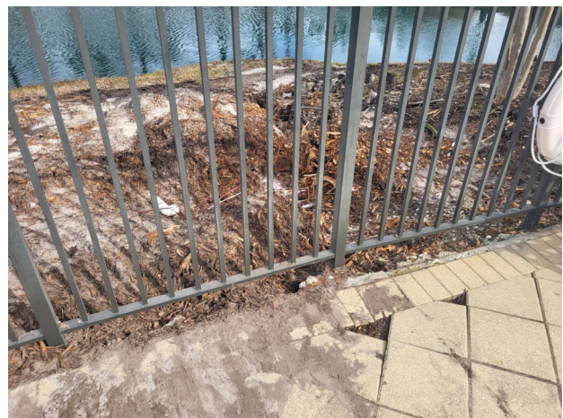
Washout from Cypress Roots
