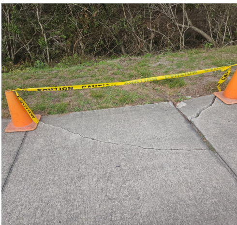
Sidewalk Collapsed On Longleaf Pkwy.
