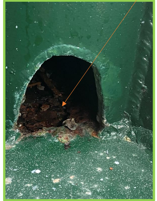
Rust Appearing from out the Drain Ports:
